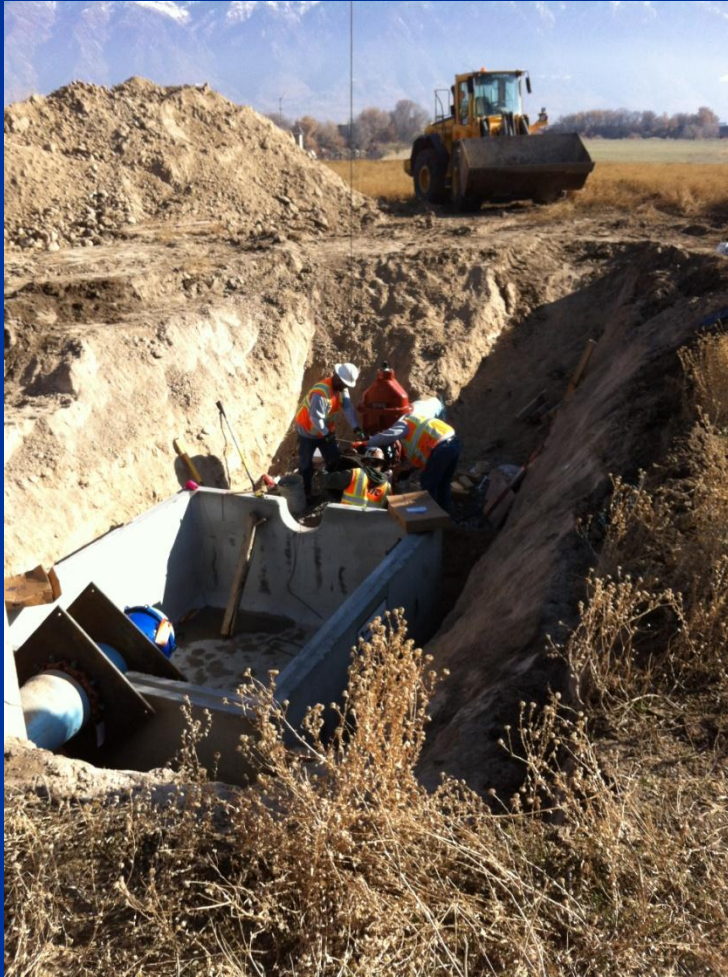
Wakegan Sewer Test Vault
