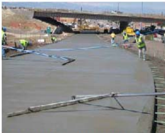
Crews pave eastbound Arapahoe Road in concrete in preparation for opening the new ramp to northbound Parker Road.
