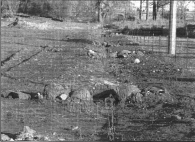
■ Onsite materials such as large rock (6" diameter or greater) may be placed in flow path to reduce velocity and erosion.
