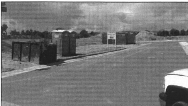
■ Construction sites must have waste containment facilities such as dumpsters, portable toilets and concrete washout areas.
