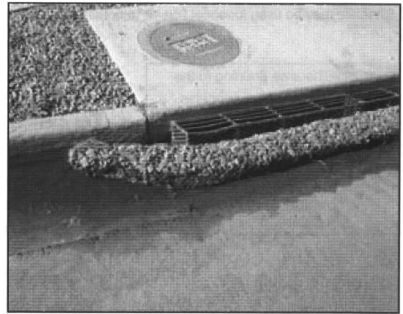
■ Effective inlet protection, such as a rock barrier, keeps sediment out of storm drains.
